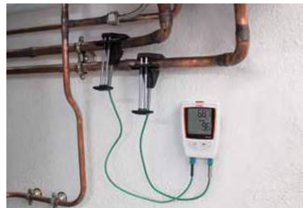
KTT 220 equipped with two clipped thermocouple sensors to control the domestic hot water network (DHW), mounted onto a wall plate
