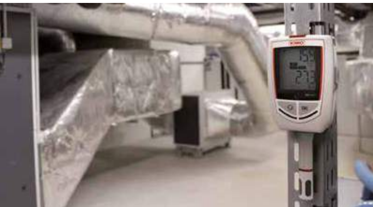
Magnetised KH 220 in the air conditioning room of an industrial facility
